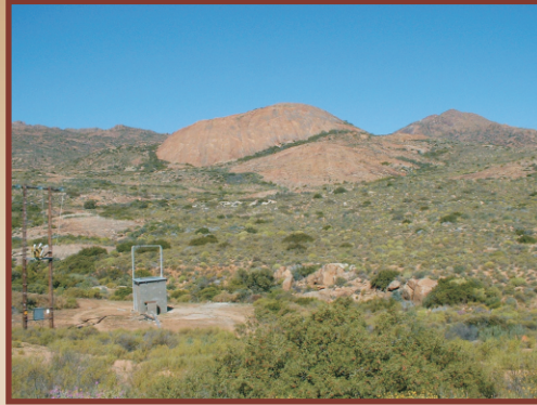
Pump house for the injection and abstraction borehole
