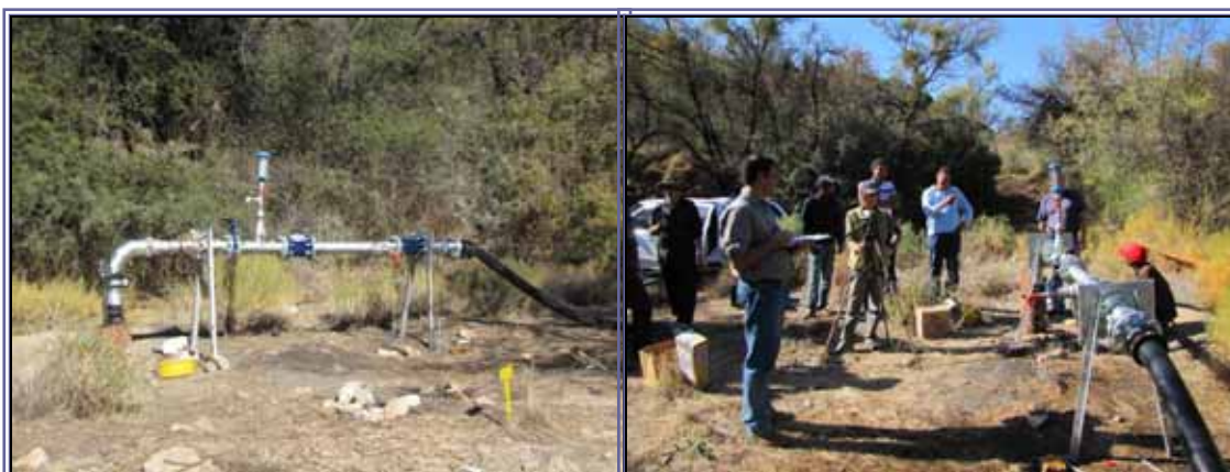
PHOTO 1 & 2: THE BOREHOLE INJECTION RIG USED FOR THE PRINCE ALBERT ARTIFICIAL RECHARGE TESTS
