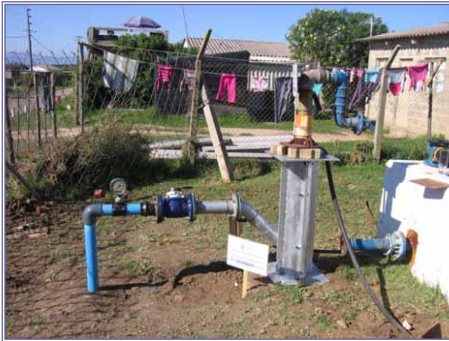
PHOTO 3.1 BH 6 CONVERTED TO AN INJECTION BOREHOLE FOR CONDUCTING ARTIFICIAL RECHARGE TESTS
